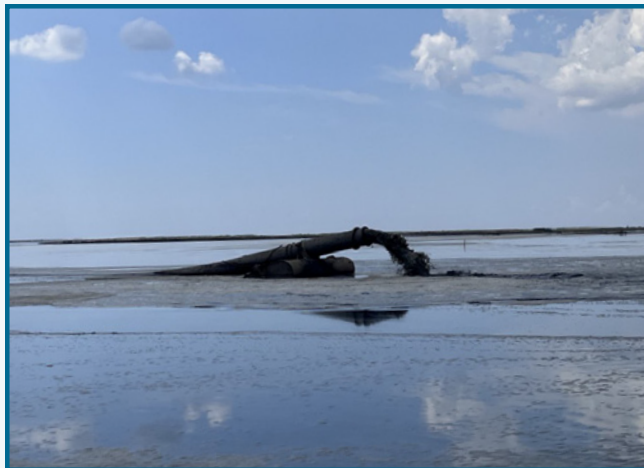
Slurry discharging into containment area. Sediment from slurry will settle and create land while remaining water will leave the site through a box weir.
