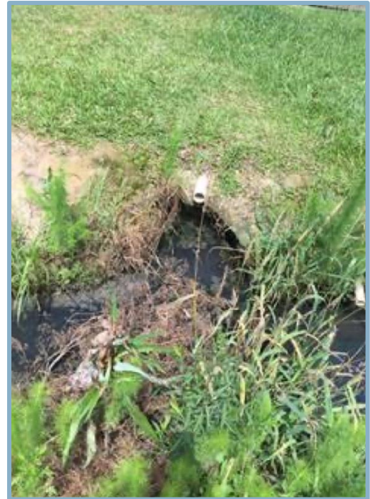
Fig 1. Ditch in front of home polluted due to home waste system not working
