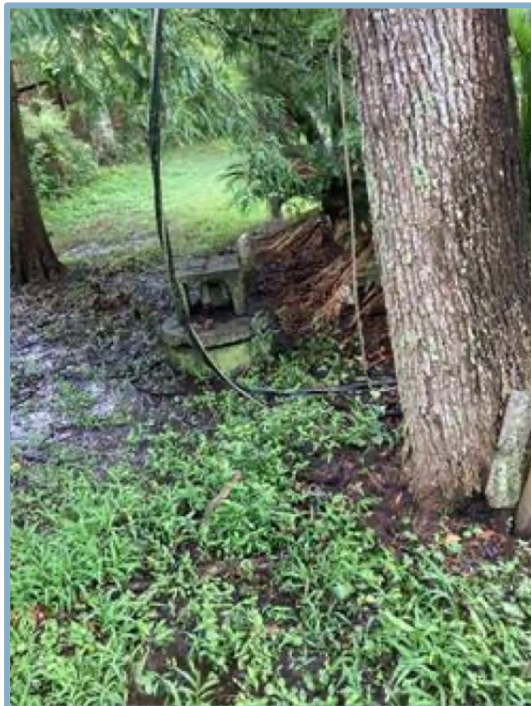
Fig 2. Sewage overflowing from an improperly managed home waste system
