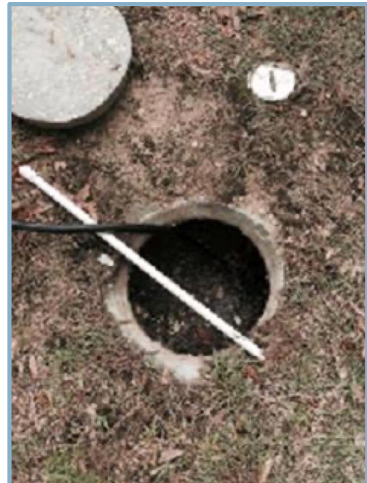
Fig 3. Home waste tank needing to be pumped out due to aerator not working for several years
