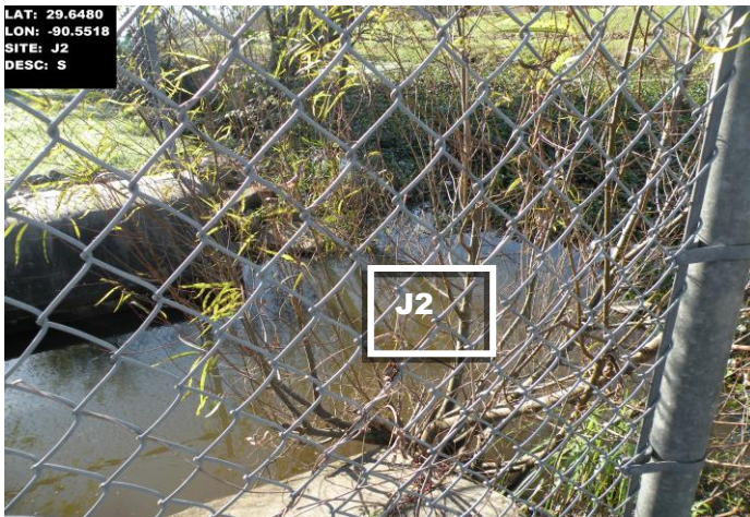
*J2 -Large cement ditch draining all of Lockport Heights which is not on city sewerage into the 40A canal “Hot Spot”
