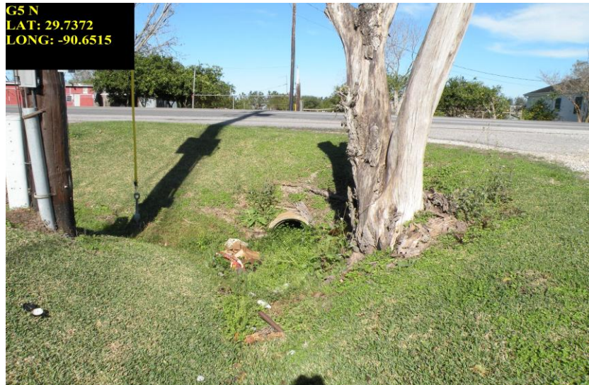
G5 Culvert at Plaisance Dr., N. Raceland (Culvert runs under LA Hwy1 to Bayou)
