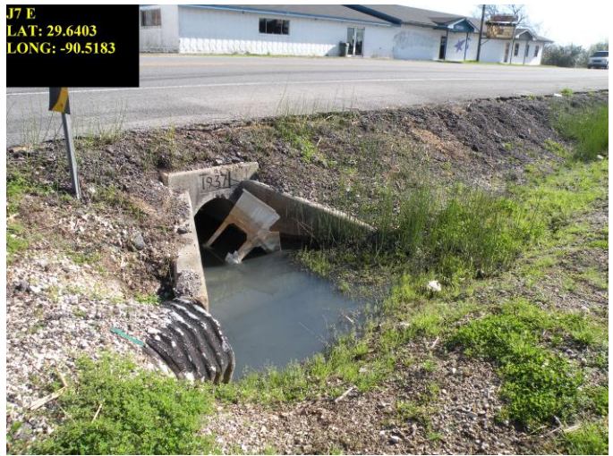
*J7 Culvert from Hwy 1 to B. Lafourche at Frank’s Store parking lot, Lockport (“Hot Spot”)
