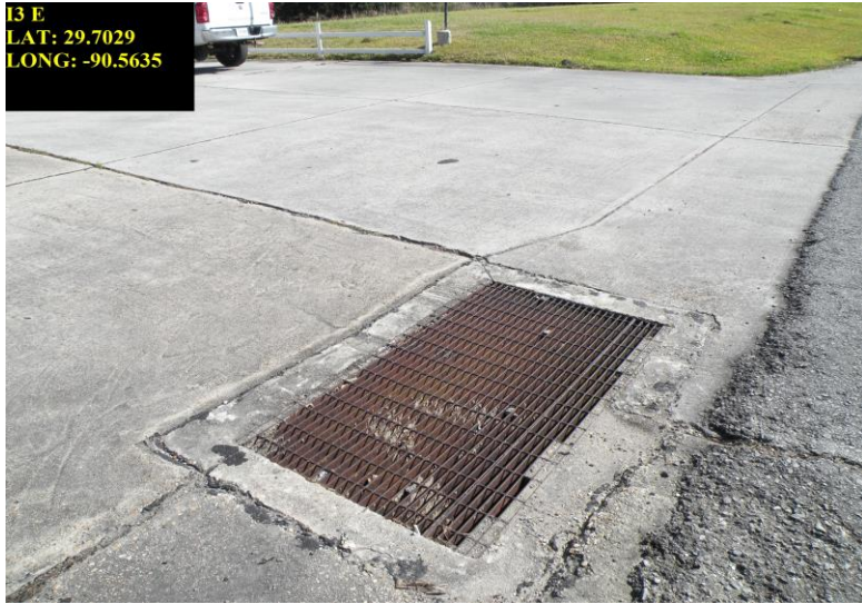
I2 Catch Basin on Hwy 1 at Acadia Road bayou side in gas station lot
