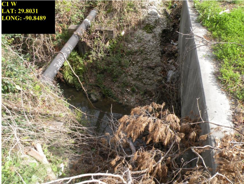
*C1 Abby Canal draining under Hwy 308 "Hot Spot"
