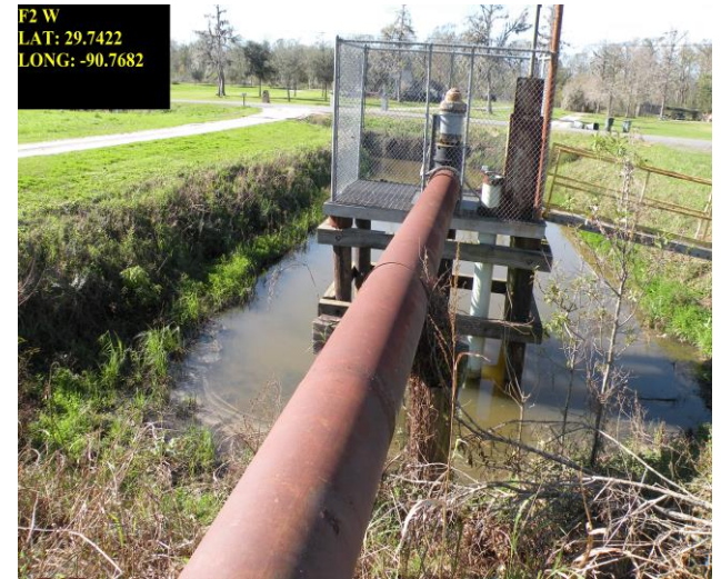
F2 Pump station from drainage ditch on Lefort Rd to 40A Canal
