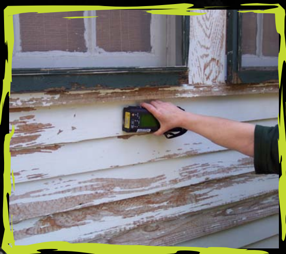
A site inspection being conducted by LDEQ staff, using the Nitron XRF to test for lead content of the paint.
