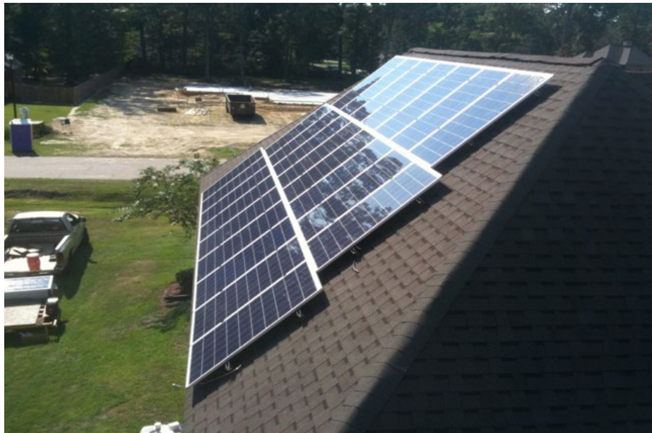
Solar panels installed on a residence by Gulf South Solar
