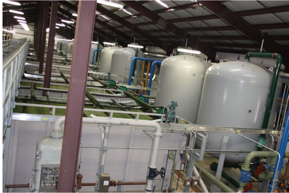
Dissolved Oxygen containers at the new West Monroe Waste Treatment plant
