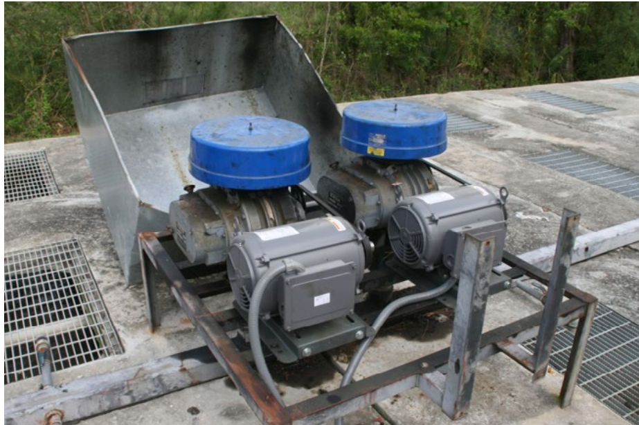
Aeration pumps situated above individual treatment cells of a waste water treatment system
