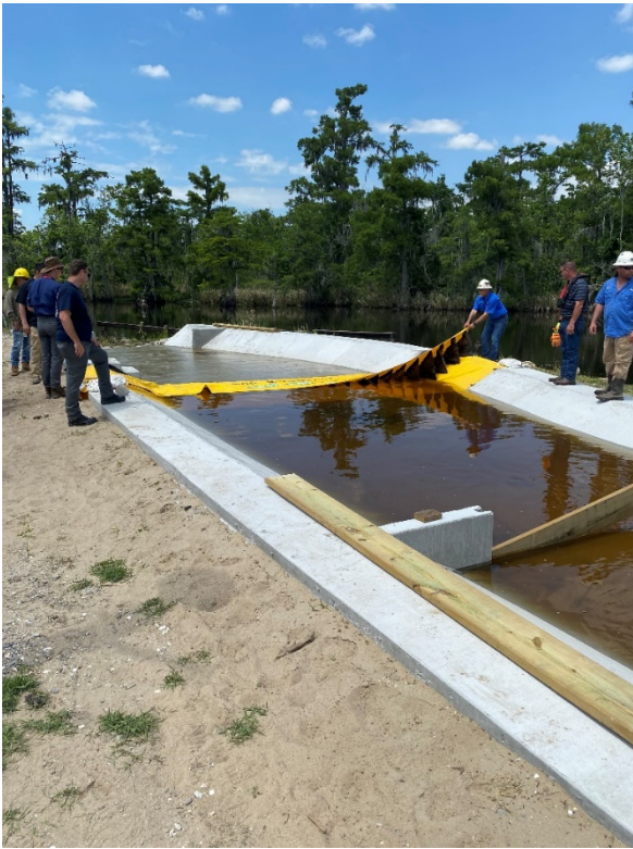
Staff install a dam during simulation of a spill on the concrete river model
